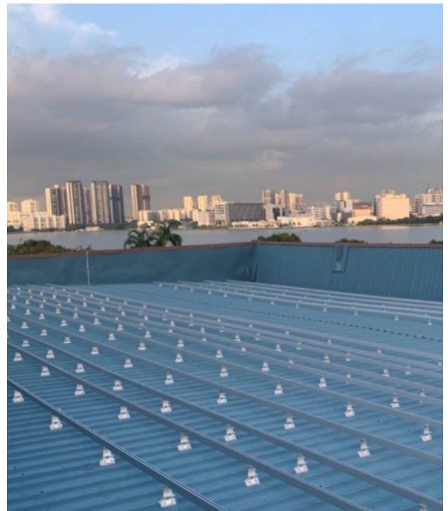
The beginning of the PV System installation process, with solar panel mounts successfully installed.
